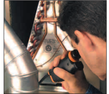
Inspecting a hard to reach point in a heating system
